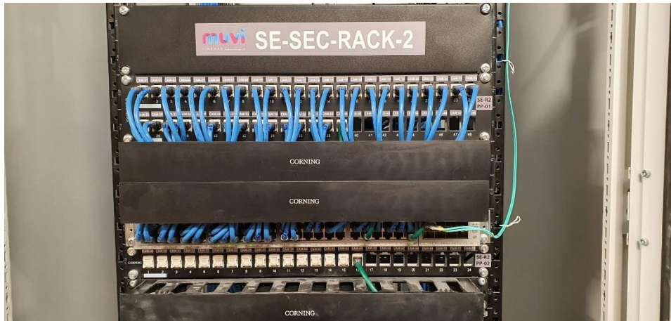
MUVI Cinema AlNakeel Mall, Riyadh. (Data Center)
