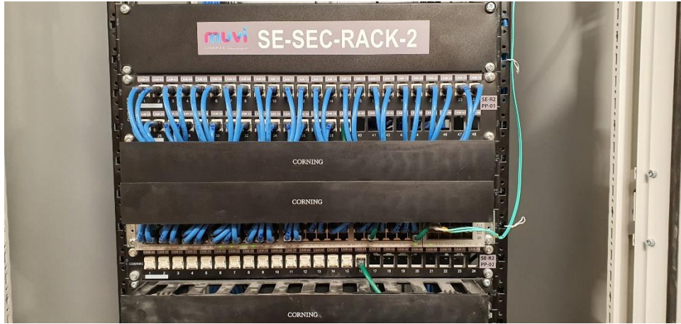
MUVI Cinema AlNakeel Mall, Riyadh. (Data Center)
